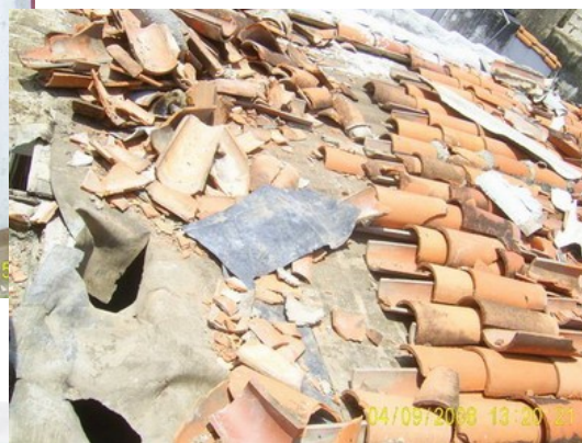
Here are Pictures of some of the damage done by Gustov.
